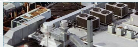
High performance HVAC controls
